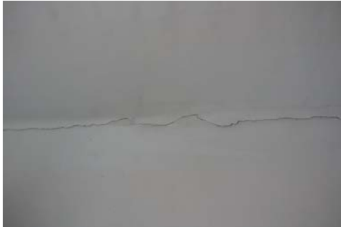
Sprekker i himlingsoverganger
