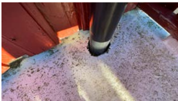
Fare for vanninntrengning.
