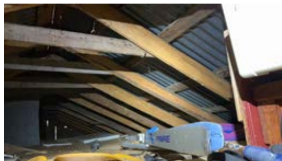
Manglende undertak under taktekking.
