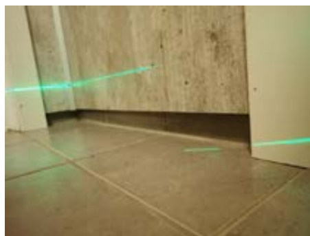
Mangelfull tetting under veggplatene
