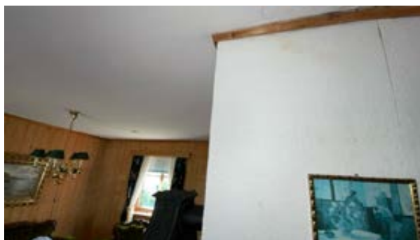
Riss i overgan pipe/brannmur.
