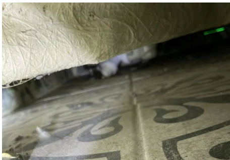
Sluk under kabinett
