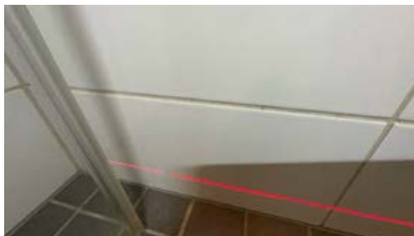
Riss i flisfuger.
