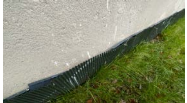
Fuksikring mangler klemlist
