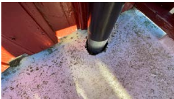
Fare for vanninntrengning.
