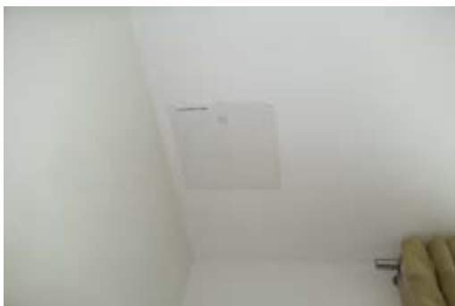
Stoppekran i himling soverom.
