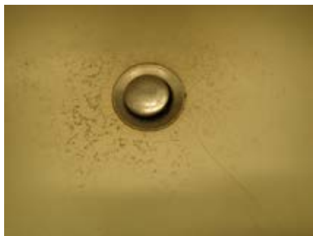
Sprekker i servant
