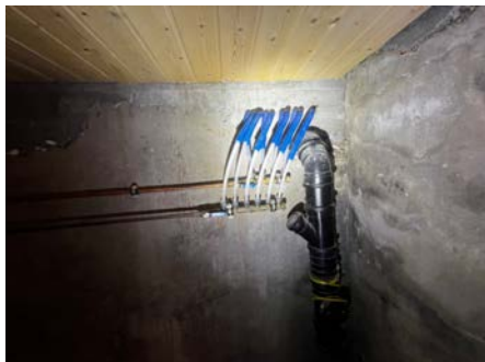
Fordelerstokk for vann.
