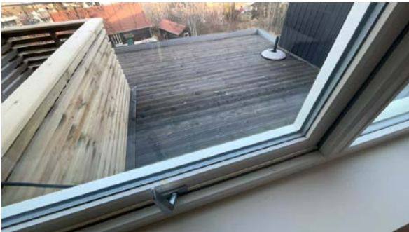
Vindu subber mot karm.
