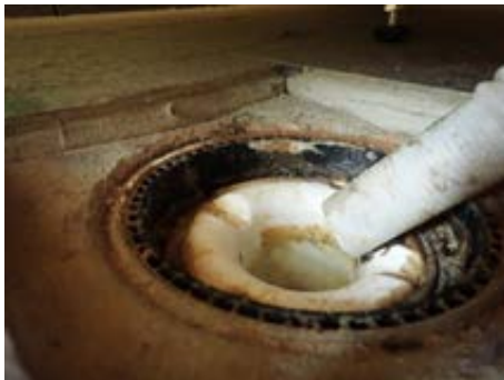
Rist mangler over sluken
