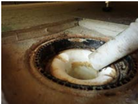
Rist mangler over sluken
