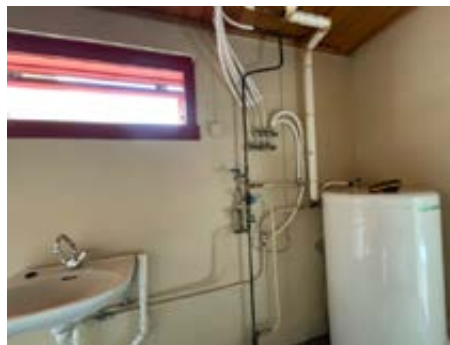
Fordelerstokk for vann.
