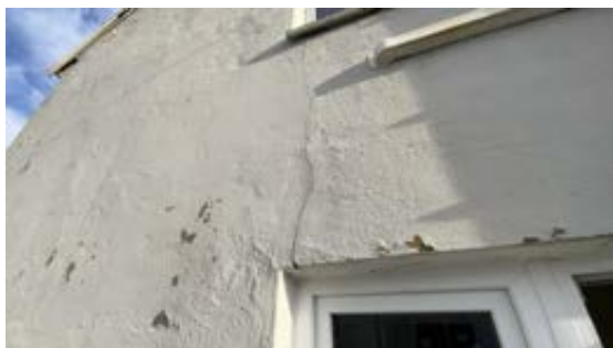
Riss/avflassing o overflatebehandling.
