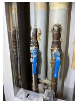
Stoppekraner bak luke i garderobe.
