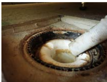
Rist mangler over sluken
