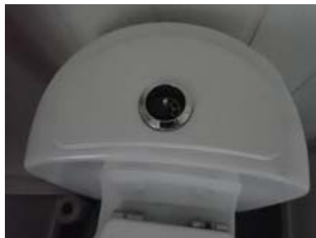
Defekt knapp for nedskylling
