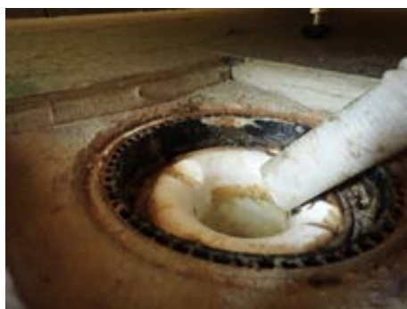
Rist mangler over sluken
