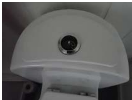
Defekt knapp for nedskylling
