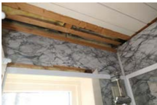
Noe manglende kledning i himling,
