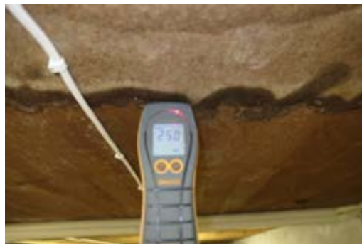
Fukt i himling.
