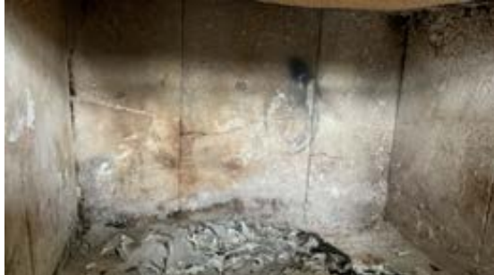
Riss/mindre sprekker i ildfast stein
