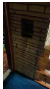
Mangler ubrennbar plate under feieluke
