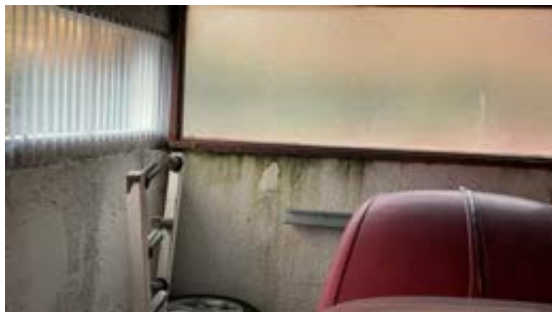
Misfarging mur bakkant
