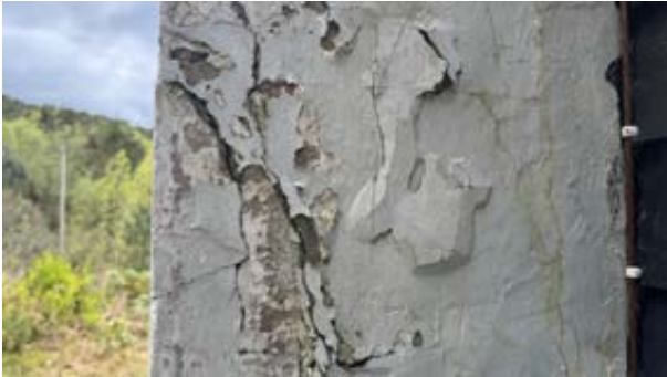
Sprekker i pipe.
